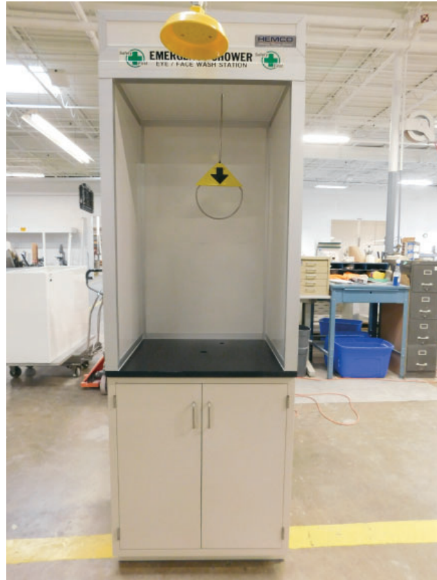
Front of safety station
